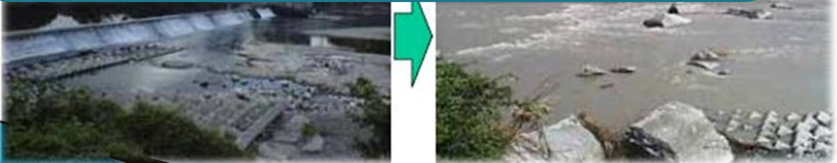
Fixed gate (60years) was collapsed by flood
